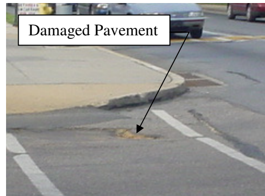
Damaged pavement in the southwest quadrant at Railroad Street and US 422.
