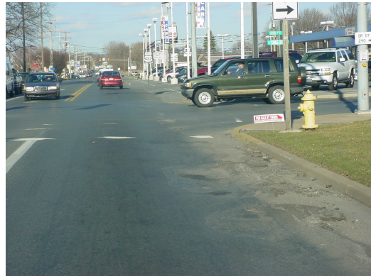
Rutting at US 422 eastbound at White Oak Street.
