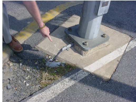
Wiring exposed in the SE quadrant at Forge Road and US 422
