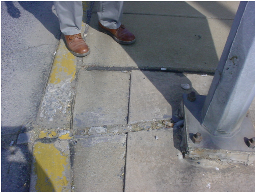
Wiring exposed in the NE quadrant at Forge Road and US 422
